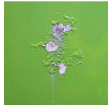
Paint damage caused by damage to the inside walls
