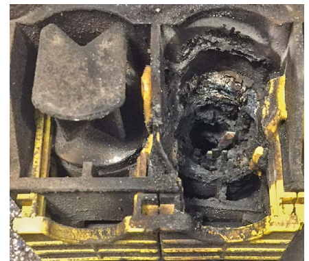
Result: as a result of moisture/poor connections, the connections of the EBS modulator can be burned out.
